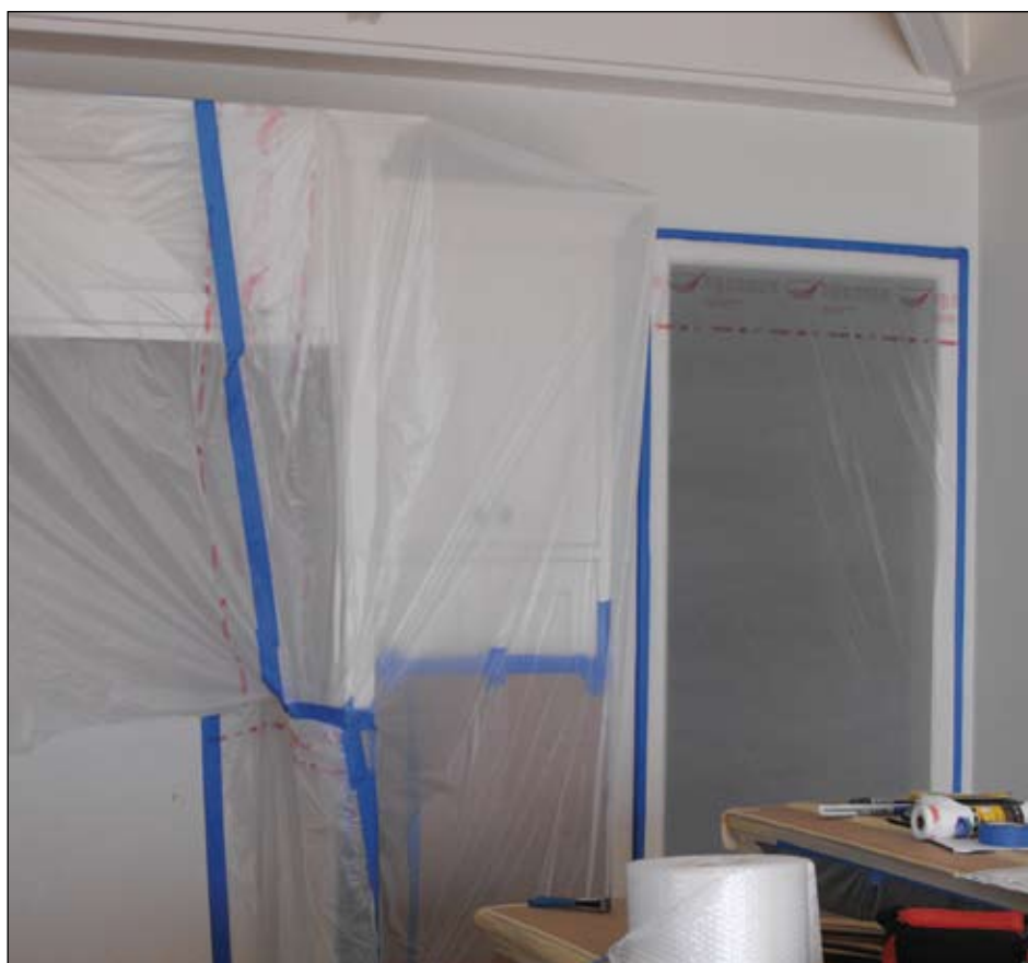
Cabinet Protection - The cabinets in this home were covered and sealed to protect them from dust, debris and the elements during renovation of that portion of the home.
