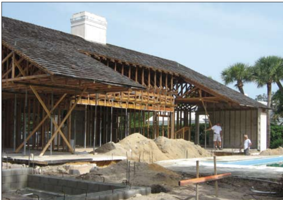
Minton before - Demolition of a home in John's Island where roof is still intact but walls and interior of the house were completely gutted.
